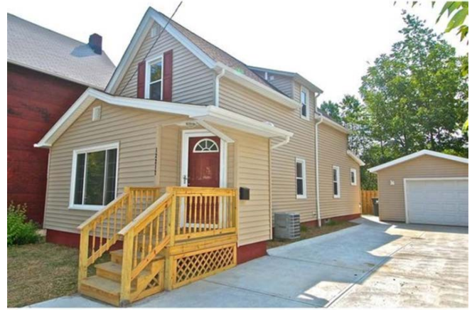
Plover Avenue rehab: exterior siding, new front steps, interior renovations, driveway, and garage.
