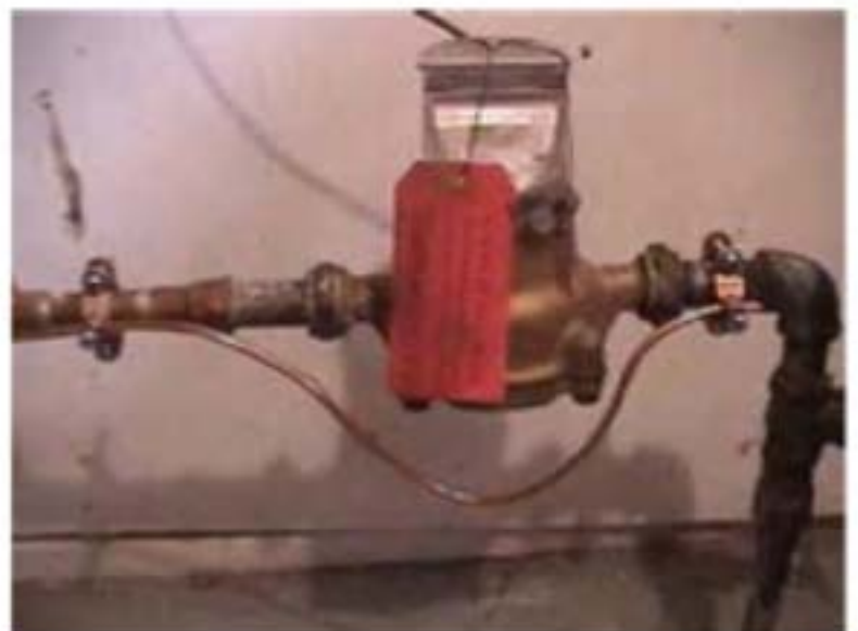
Typical Water Meter
