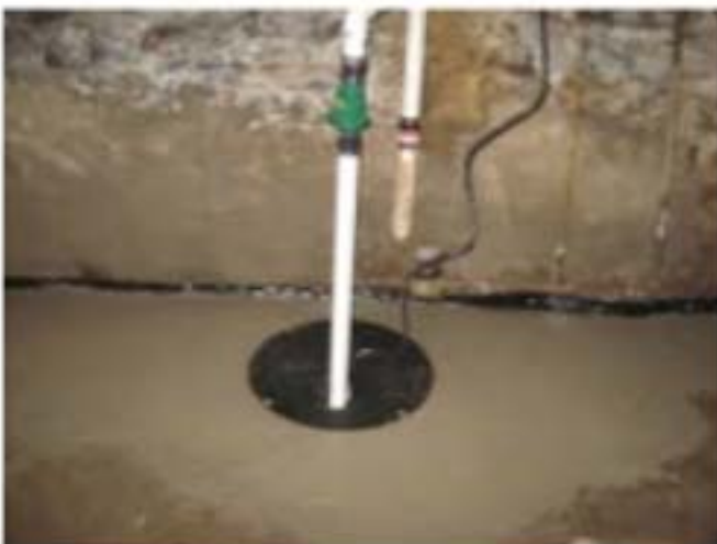
Typical Basement Sump Pit/Pump
